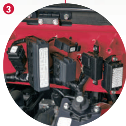
Electrical fuse box and relays
